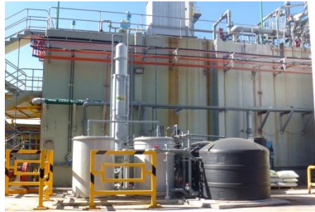
Scrubber and compost biofilter for odor control
