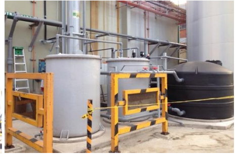
Scrubber and compost biofilter for odor control
